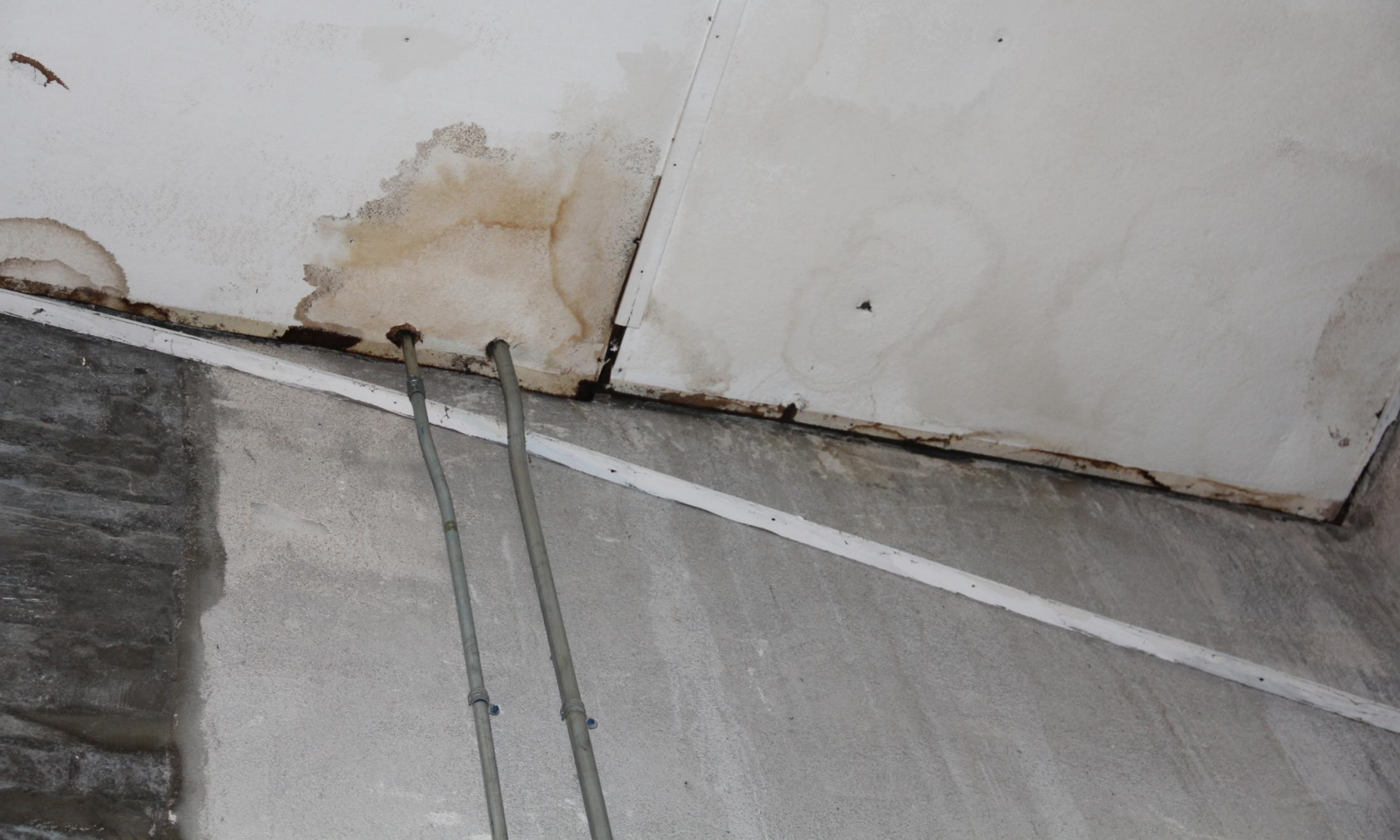
Water damage in bell tower
