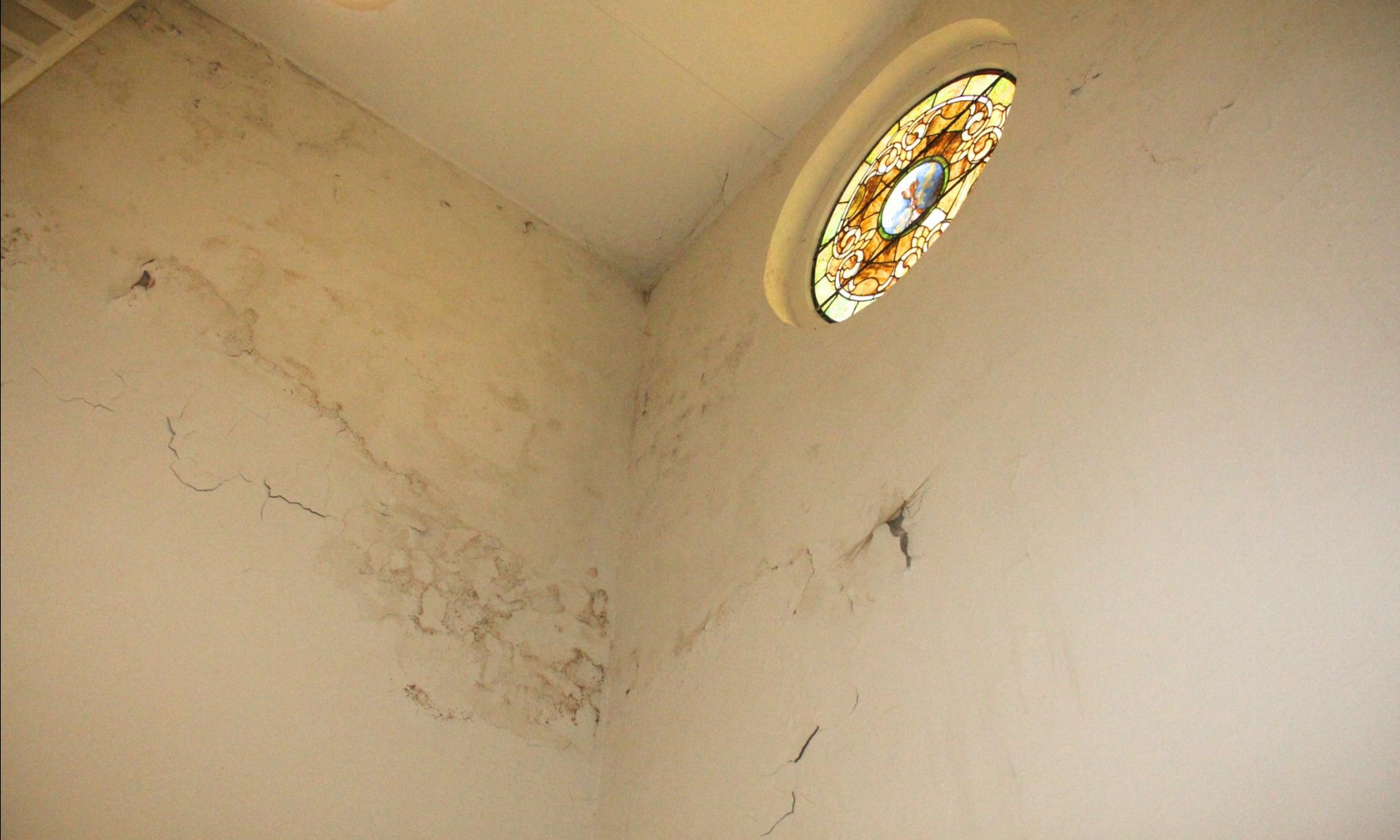
Water damage in stairwell (north tower)
