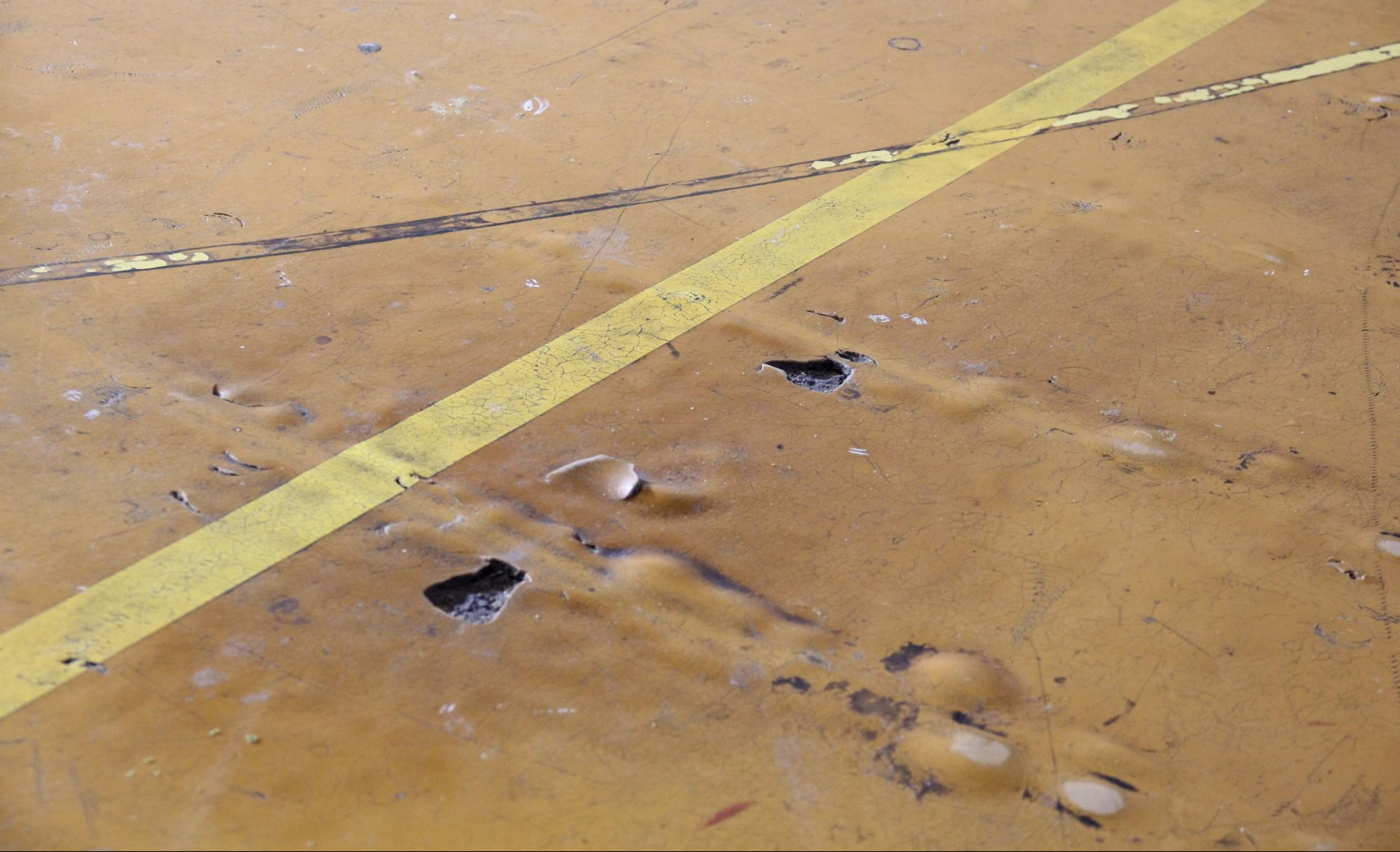
Damage to gym floor
