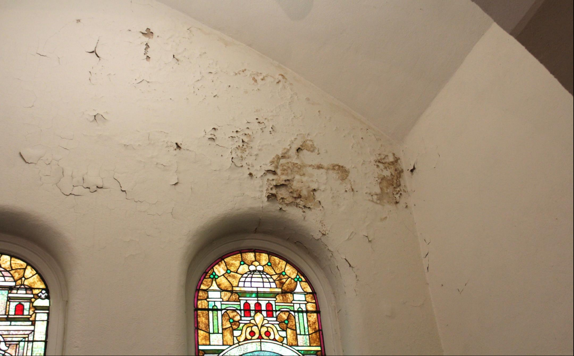
Water damage in choir loft
