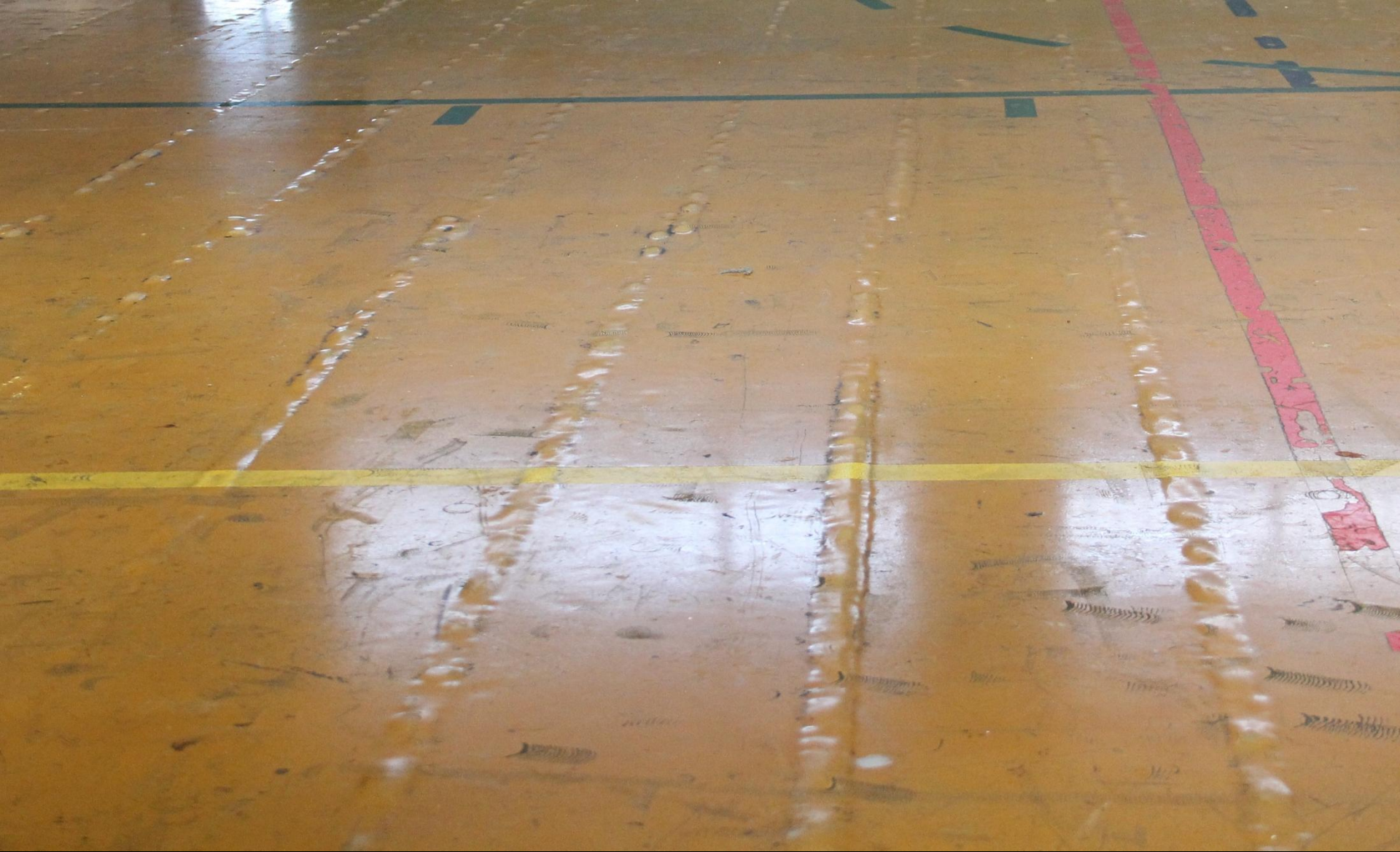
Damage to gym floor
