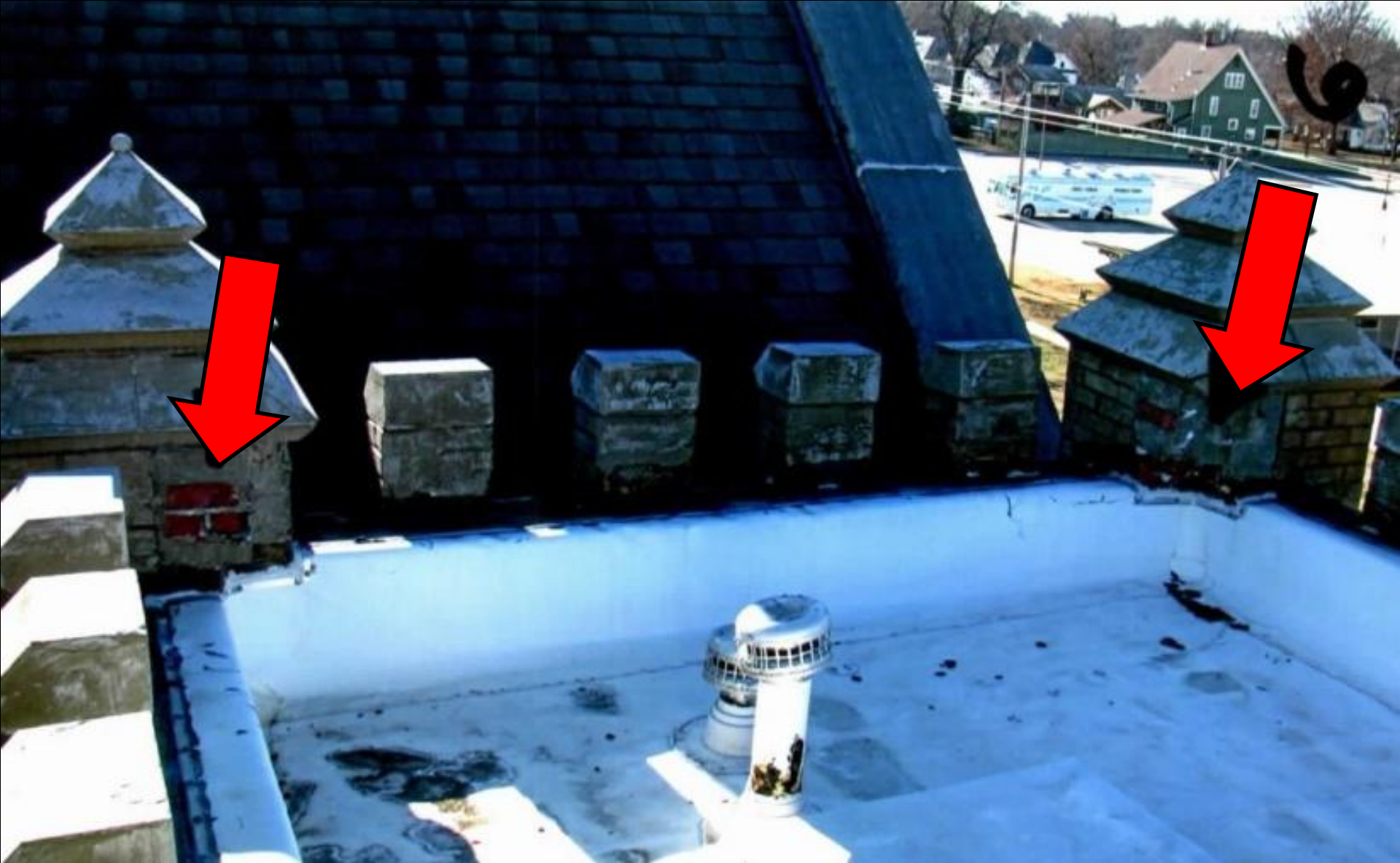
Damaged brick merlons
