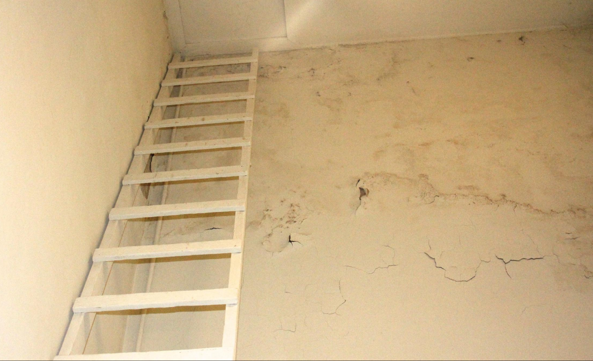
Water damage in stairwell (north tower)
