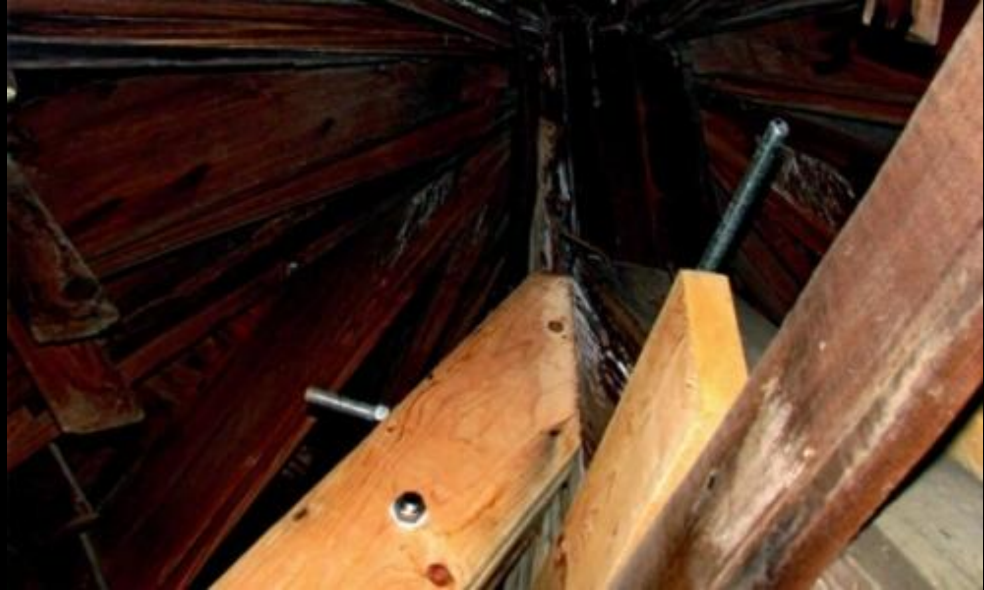
Water damage inside dome
