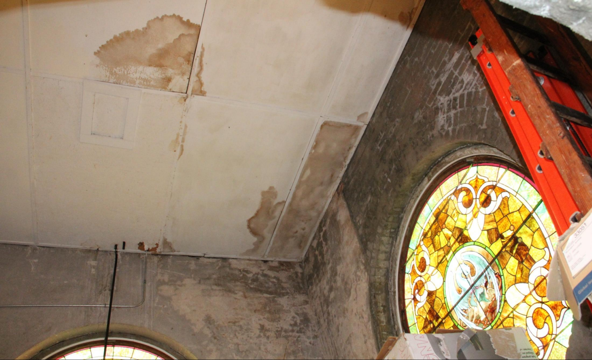
Water damage in bell tower
