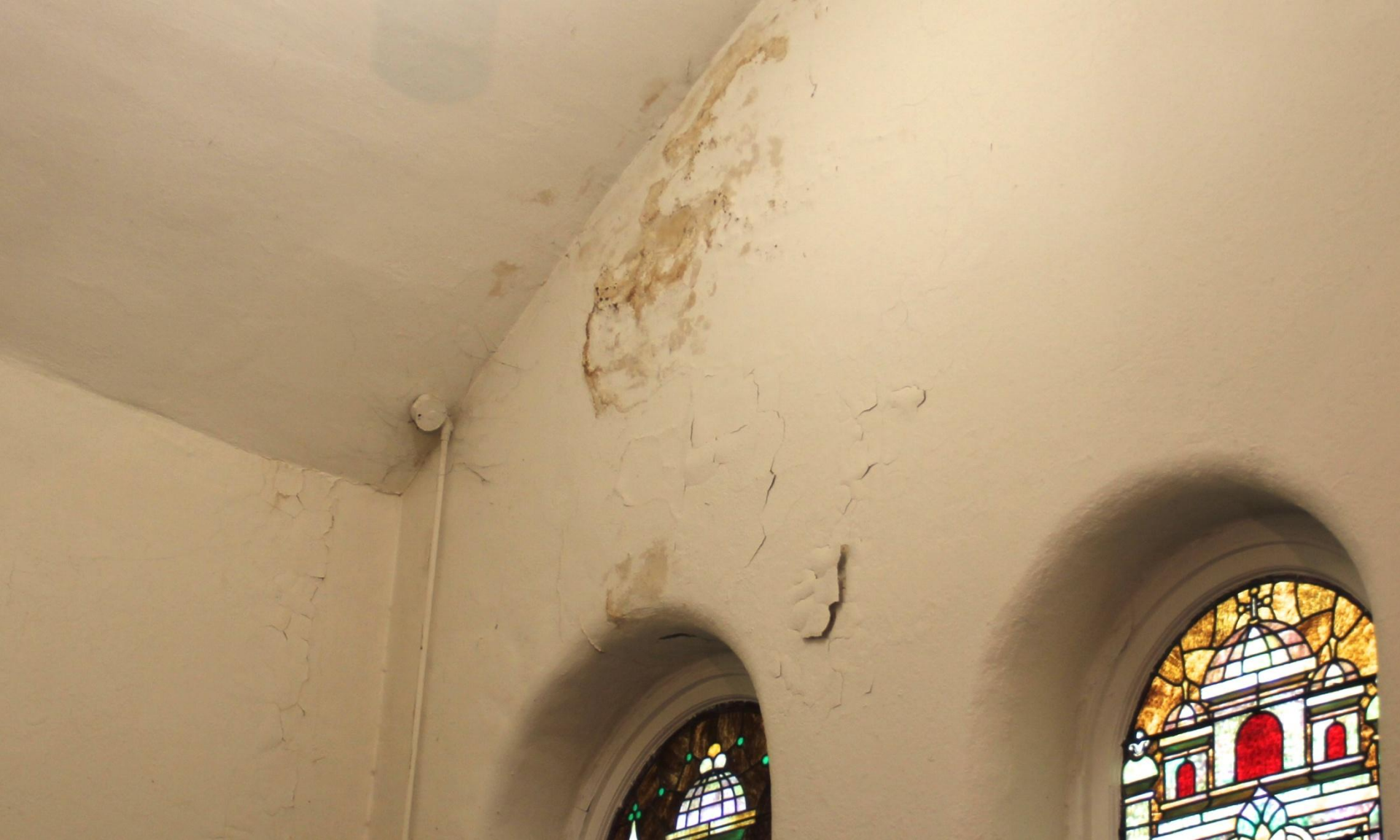
Water damage in choir loft
